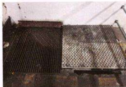
OGT – OIL & GREASE TRAP CHAMBER
