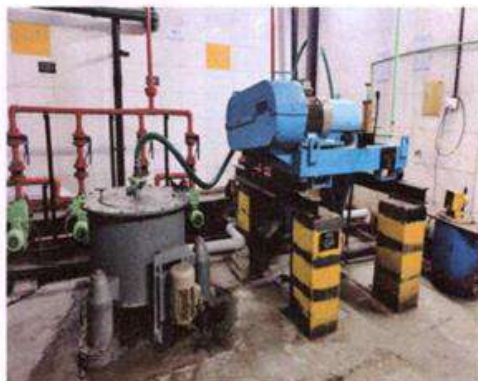
CENTRIFUGE FOR SLUDGE PROCESS
