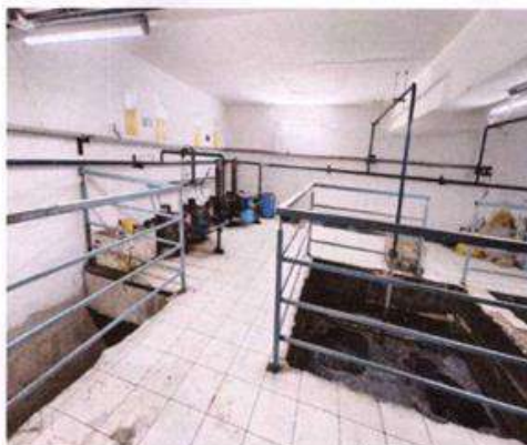
PLANT ROOM SBR TANK EQUALIZATION TANK AND AIR BLOWER
